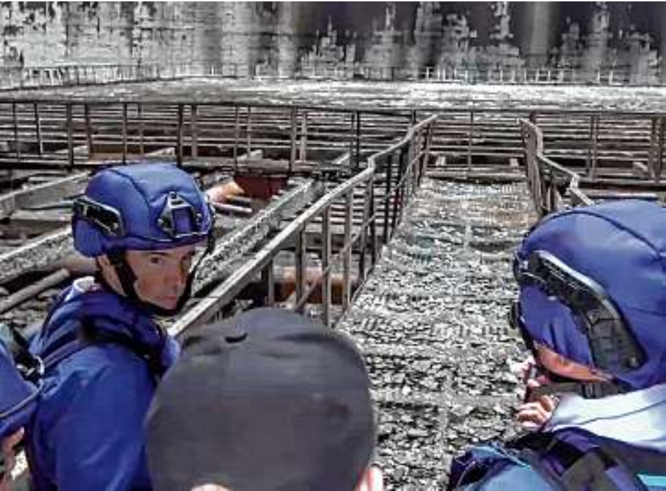
International officials examine the damaged cooling system of the Zaporizhzhia power plant.
