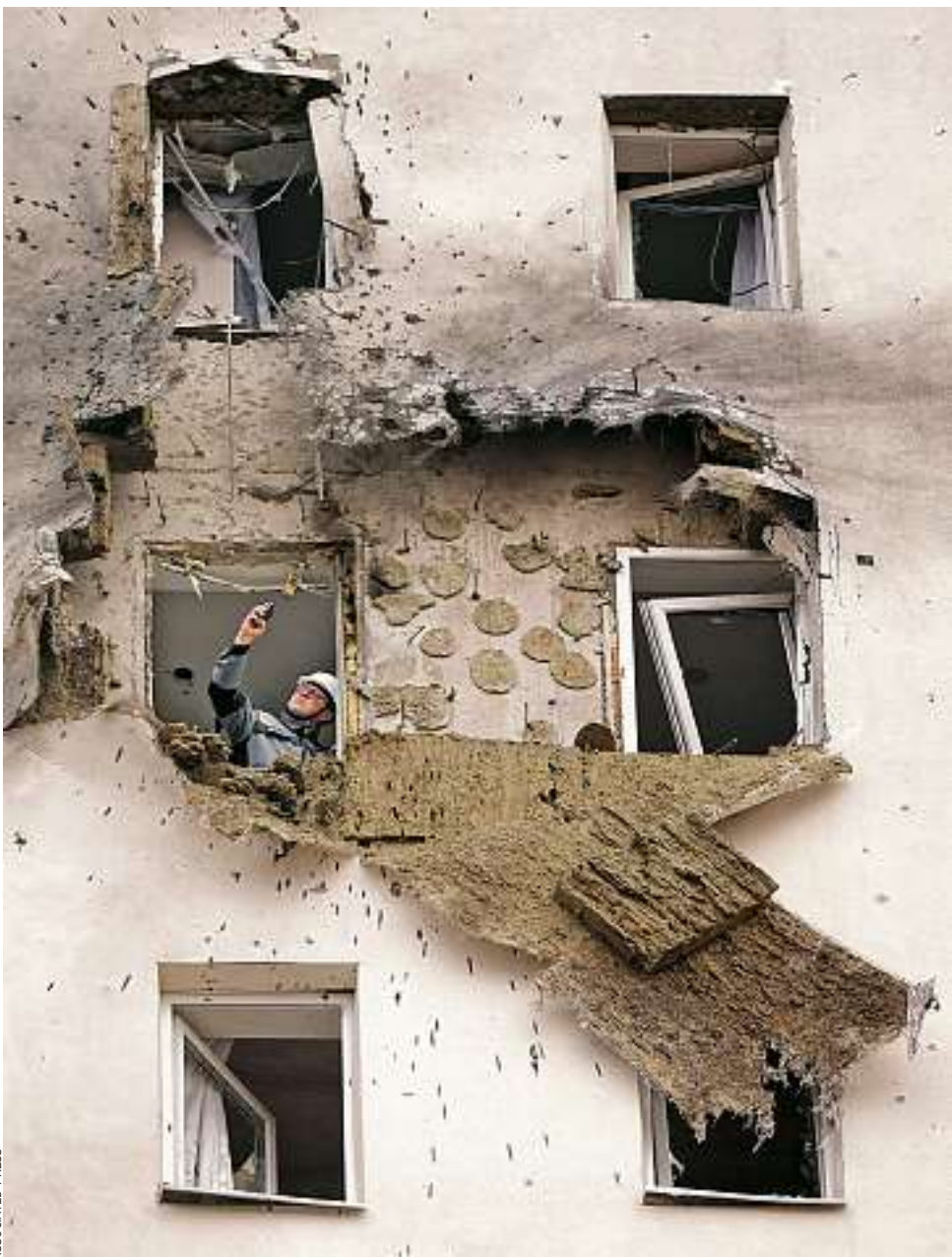
Before Ukraine agreed to a 30-day cease-fire, it launched its biggest drone attack yet against Moscow. An investigator examined apartment building damage on Tuesday. A6
