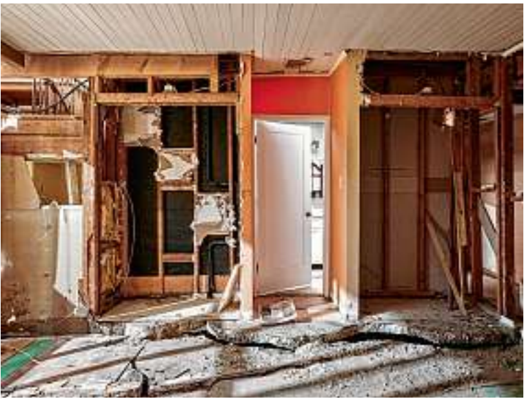
Despite significant damage, Sallie and John Reeves still live in this Portuguese Bend house where they’ve lived for 41 years.
